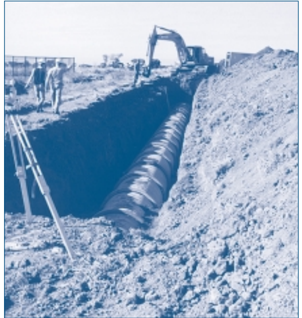
Whilst much of the Werribee Irrigation District is serviced with concrete lined channels, a steady program has been underway in recent years to replace these, when life expired, with pipeline. Although pipelining is a more expensive capital cost, the benefits in terms of both longer life and lower maintenance costs, as well as the potential for saving water, are sufficiently attractive to warrant this additional investment. Also, as the urban areas of Werribee and the City of Wyndham grow, it is essential that the risk posed by open channels - especially the Main Channel through which water can flow at quite high speeds - is eliminated. In this situation, pipelining is funded jointly by SRW and the developers of the new estates.
