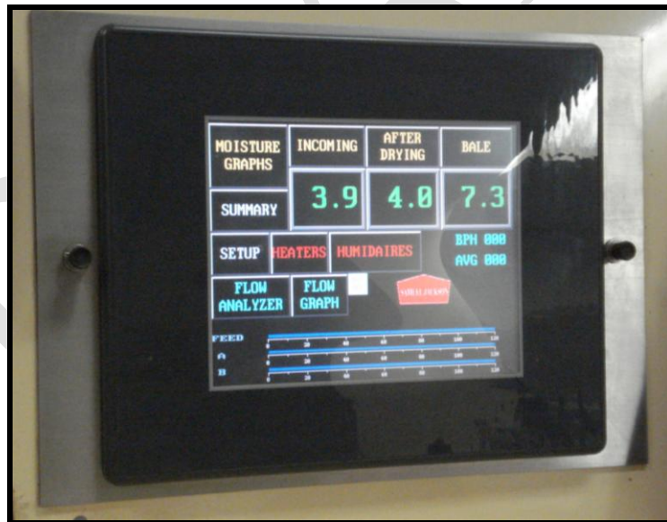
Figure 6.2: Moisture mirror in the control room
