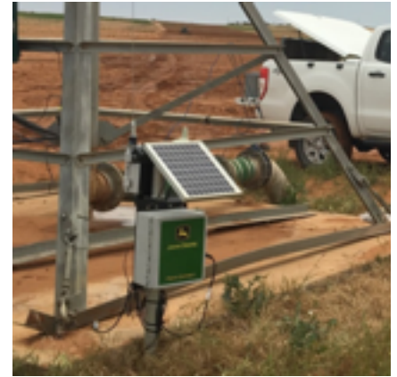
Figure 2. Central control box.
