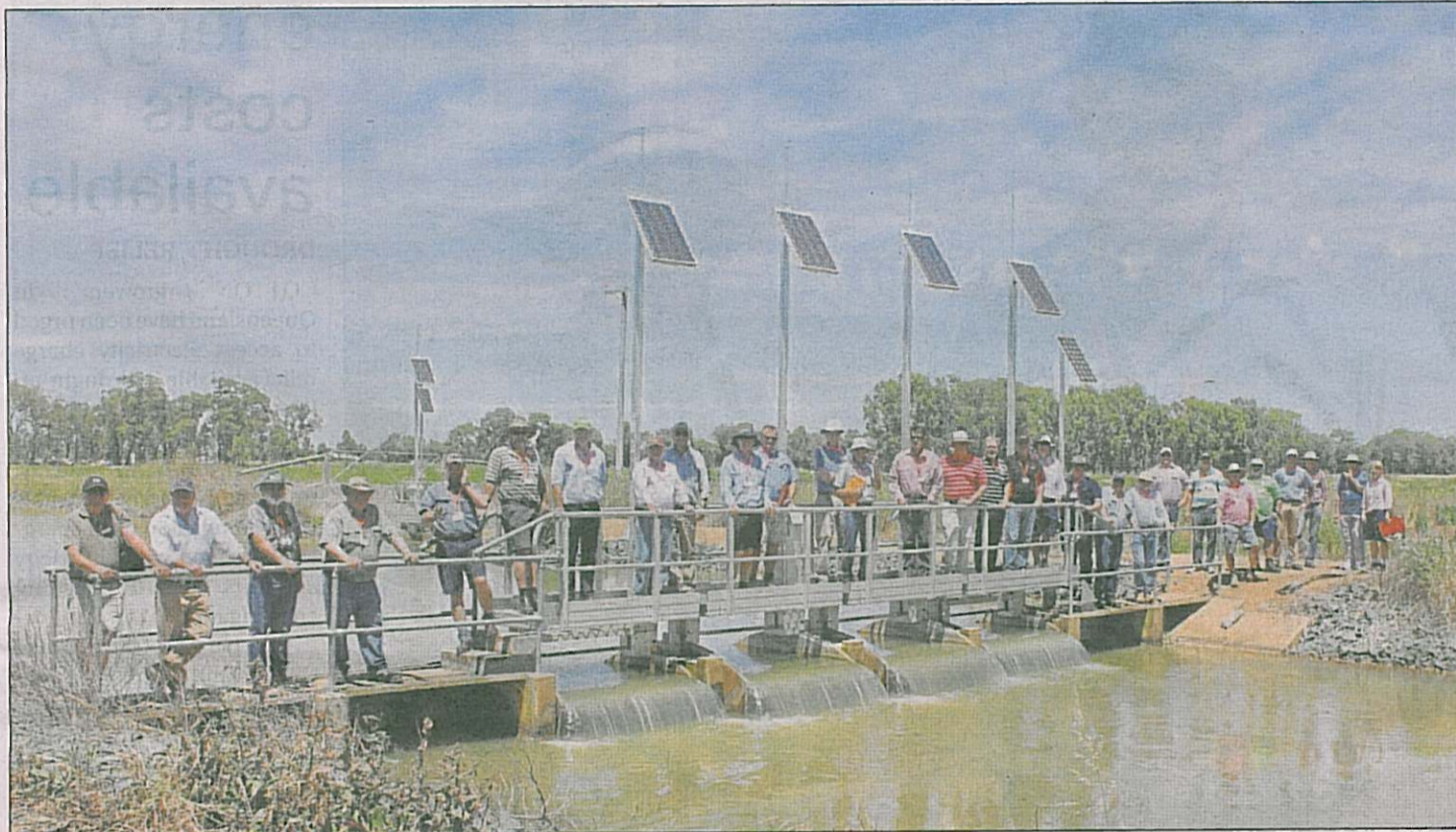
Automating in action. An automated gate outside of Shepparton.
