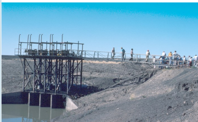
Figure 2 : Older style pump station installations in the Australian cotton industry (R.J. Smith).
