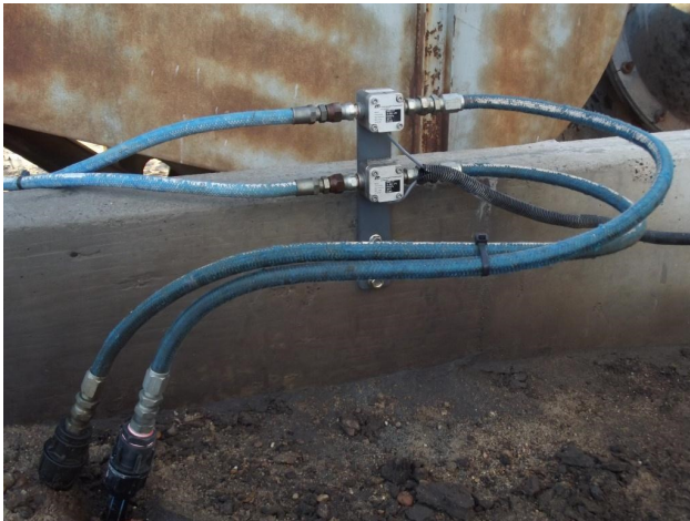
Fuel flow meters measuring diesel in-flow and return.
