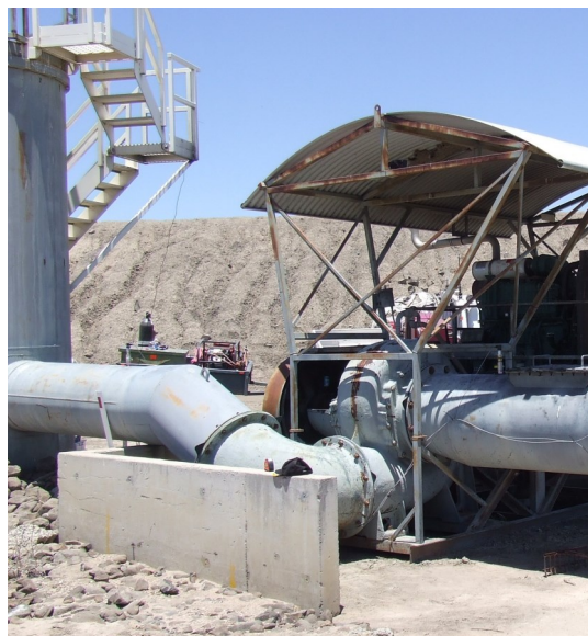
Typical lift pump station setup for a pump test
