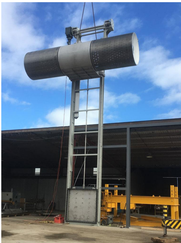
Figure 21: A T style retrievable wedge-wire self-cleaning cylinder screen in the raised position. Image reproduced with permission from AWMA https://www.awmawatercontrol.com.au/products/cylinder-screens-powered
