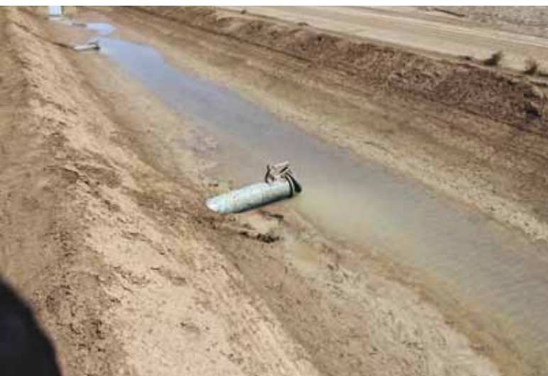
Pipe through the bank with valve mechanism.
