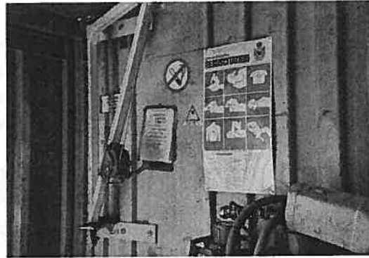
Photo 42: Inside chemical storage shed showing lifting hoist, emergency contacts, safety signage and procedures
