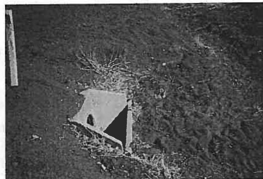
Photo 34: Concrete sills on drainage channels to prevent soil wash-off from fields
