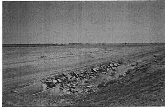
Photo 36: Area affected by salt scalds
