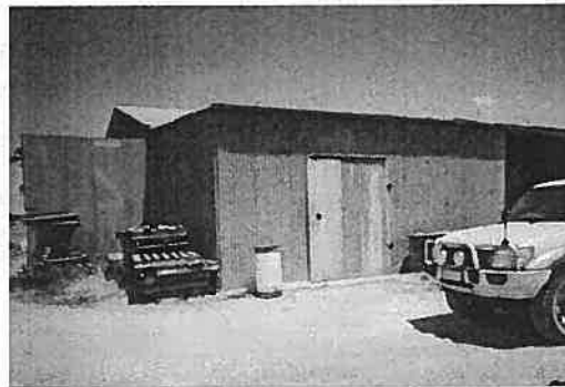
Photo 11: Non-complying chemical store - no bunding, signage or ventilation.
