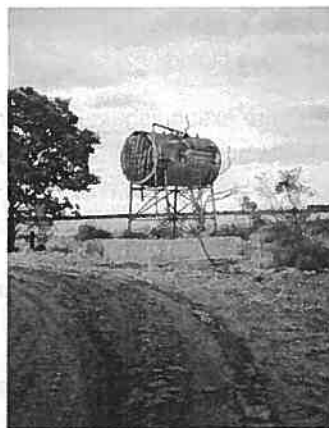
Photo 20: Bund is too close to tank
