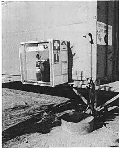
Photo 41: First aid kit, fire extinguisher, safety shower, signage at pesticide store
