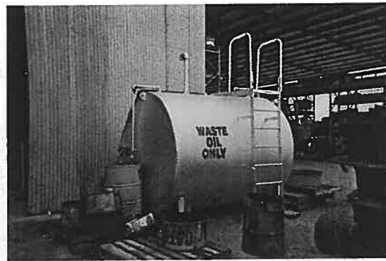
Photo 26: Waste oil collection tank
