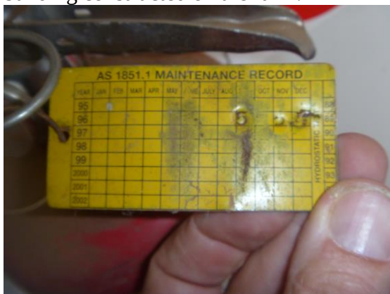
Fire extinguisher maintenance checked and updated
