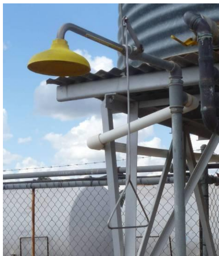
Emergency shower fixed so that water flows
