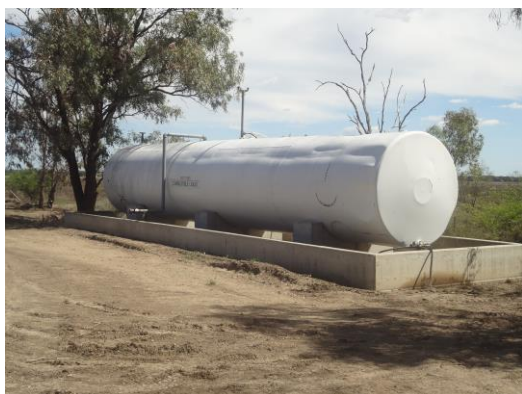
Bunded petrochemical storage
