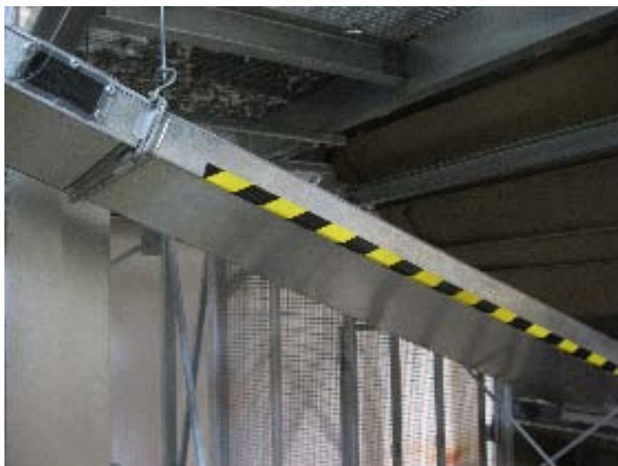
Figure 31 – Ducting (600 mm wide) between the rear of the CMSE gin stand and first lint cleaner; note no 'Super-J' bend between gin and lint cleaner
