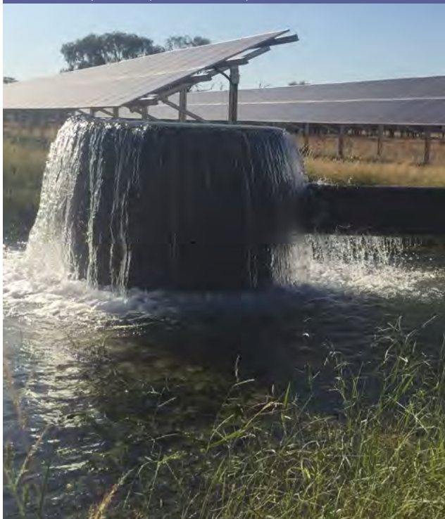
FIGURE 3: An industry first installation of a 55kw submersible pump driven by combined 100KW solar and 110kVA diesel generator at the Gill family's "Waterloo" Narromine, NSW. (Photo: Jon Welsh)
