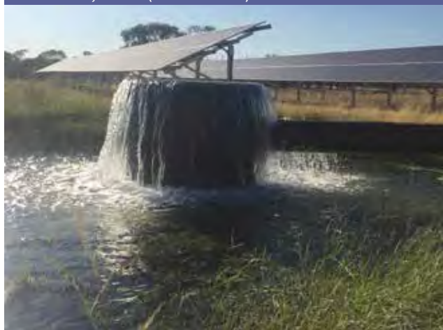
FIGURE 3: An industry first installation of a 55kw submersible pump driven by combined 100KW solar and 110kVA diesel generator at the Gill family's "Waterloo" Narromine, NSW. (Photo: Jon Welsh)
