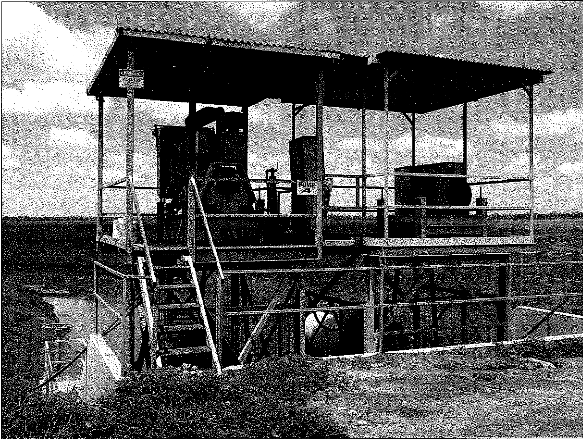
Fig8 : A comparison of performance following pump system efficiency evaluations on two pumps located side by side resulted in the operator implementing a strategy that will significantly reduce energy costs
