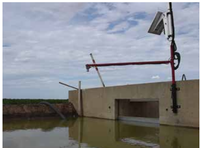
Monitoring and maintaining consistent channel head heights ensures more even siphon flow rates and more efficient irrigation. (Photo: Lou Gall, GVIA)
